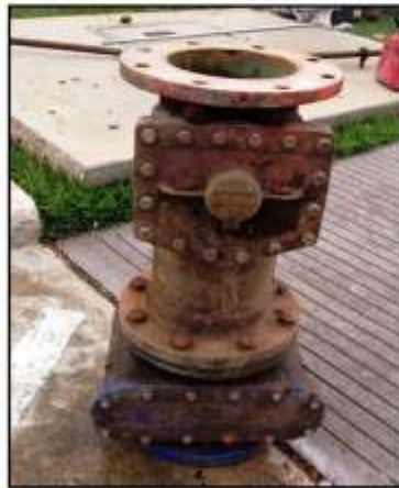
Old Meter Removed
